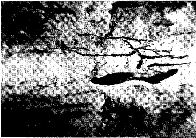
Figure 4. Detail of the defects on the outside surface of a damaged tube (Breda Institute).
